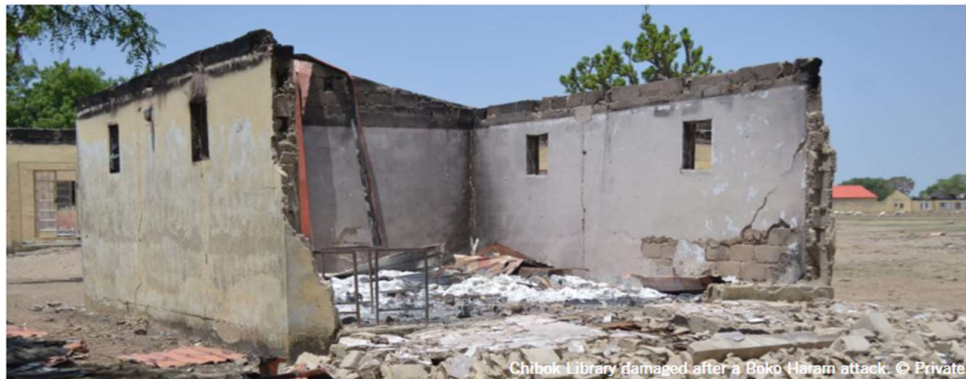
(Fig 2: A damaged Chibok Library after a Boko Haram attack (Private, as cited in Amnesty International, 2015).
