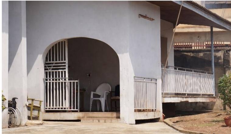
Figure 31: Entrance lack ramps, level differences are not clearly articulated
