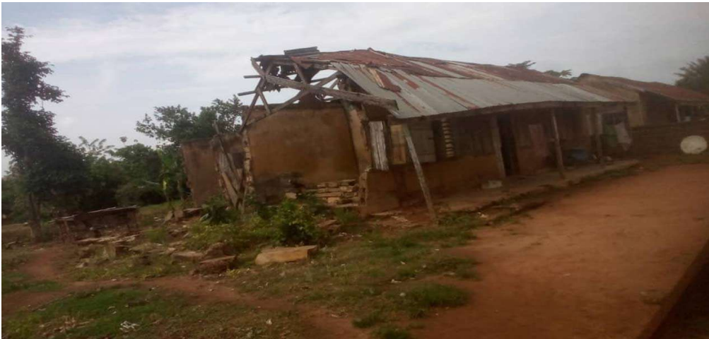
Figure 3: Deteriorated condition of infrastructure at the Akufo Farm Settlement, Ibadan, Oyo State
